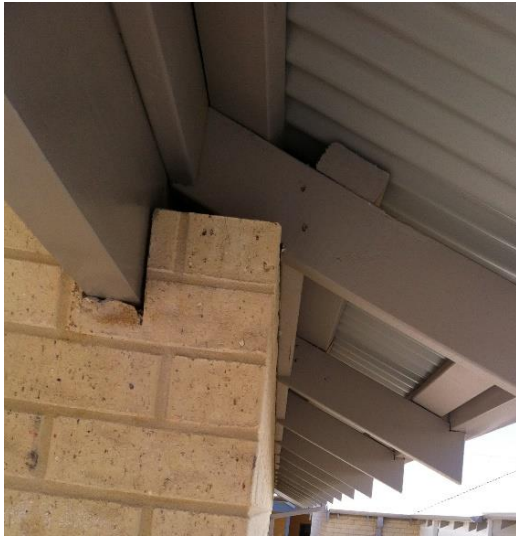
BAL construction can struggle with industry tolerance of lower standards, such as this BAL 12.5 build with gaps greater than 3mm. Credit: J de Jong
